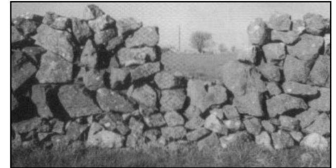
Boundary wall damaged by fox hunting - more work and liability for the farmer.
